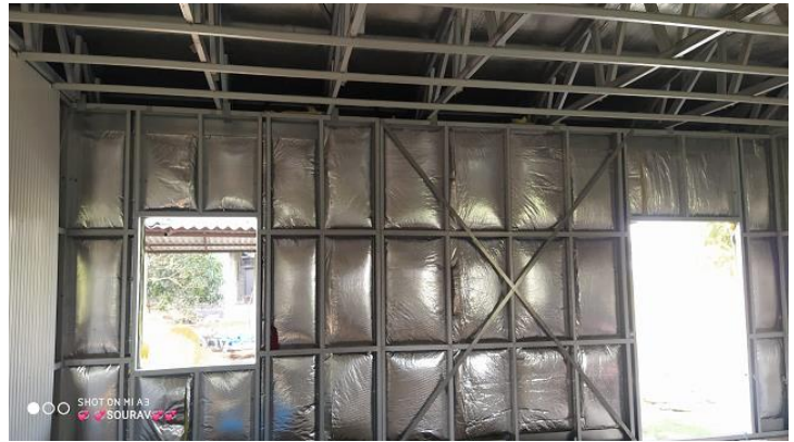
Inside of the pre-fabricated centre
