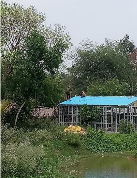
The setting up of the pre-fabricated structure at the Vidya Niketan study centre, Bamunara
