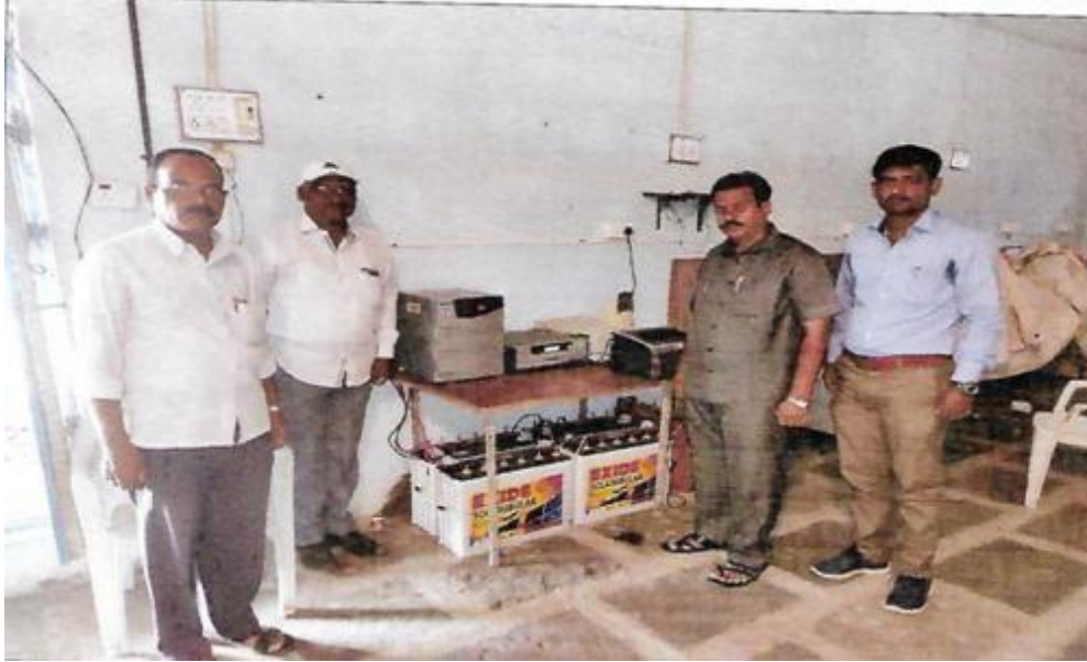
Solar panel power installation
